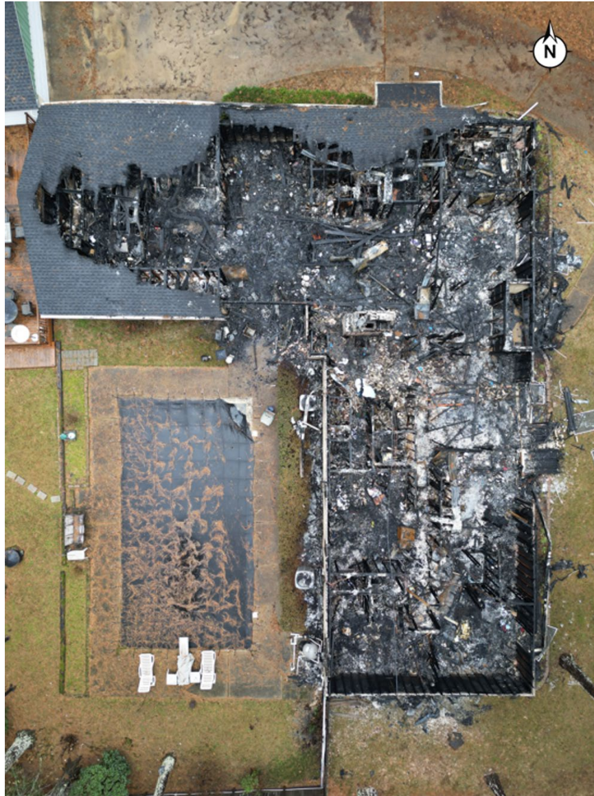
Figure 4. Aerial photograph of the Bristol Boulevard accident home after the explosion and fire. (Courtesy of Atmos.)
