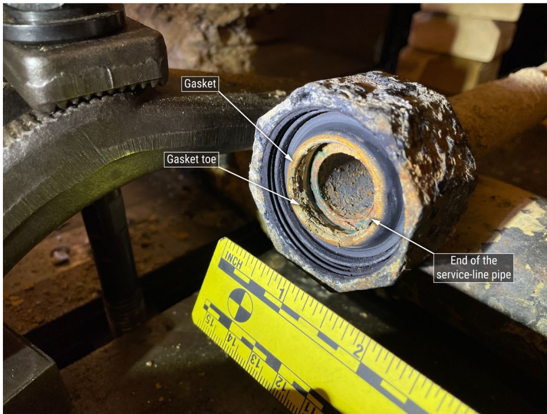
Figure 19. The Shalimar Drive service-line pipe and gasket.
