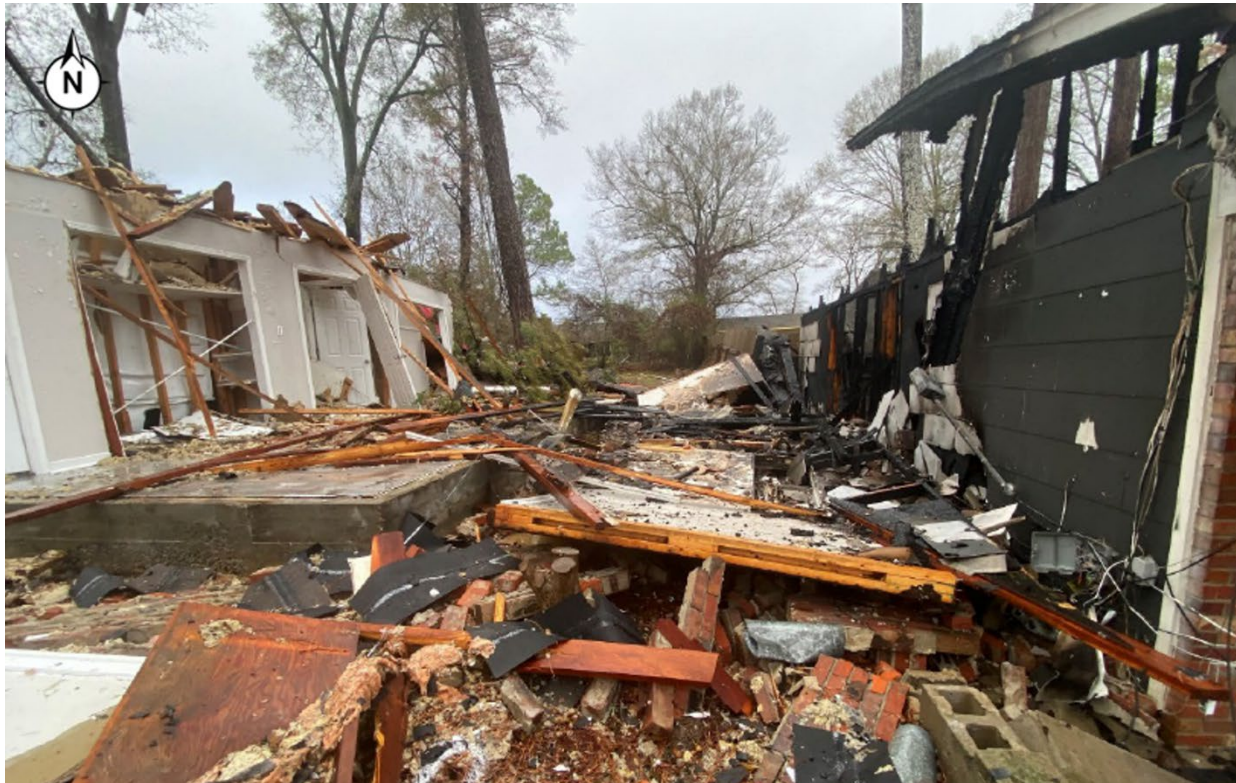
Figure 7. The Shalimar Drive accident home (left) and the Shalimar Drive affected home (right) after the explosion and fires. (Courtesy of the Mississippi Public Service Commission.)
