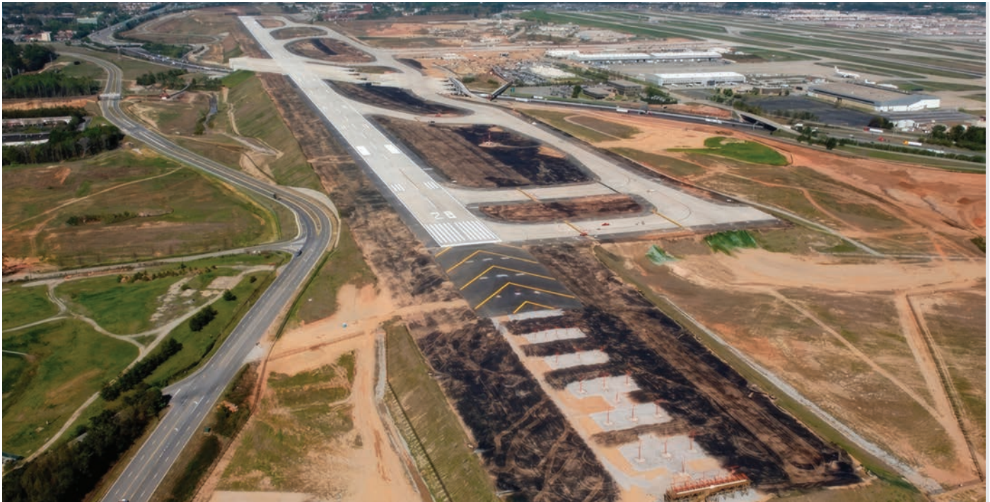
Runway construction underway at Hartsfield-Jackson Atlanta International Airport in Atlanta, GA. FAA Photo.
